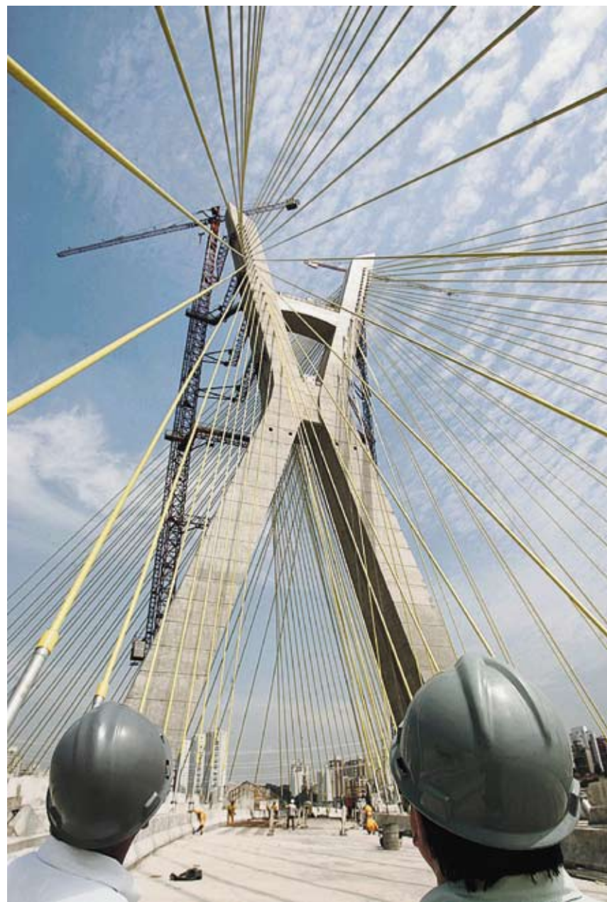
Construction of the Octavio Frias de Oliveira bridge in São Paulo Reuters
